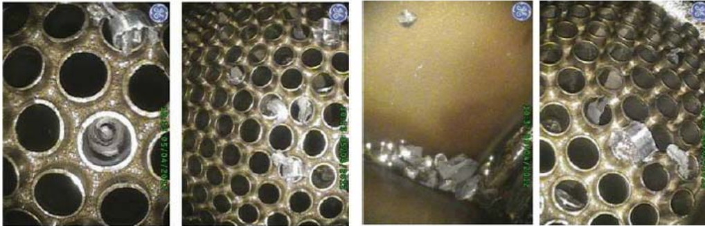
[Figure 11] Fuel/Oil Cooler Contamination
