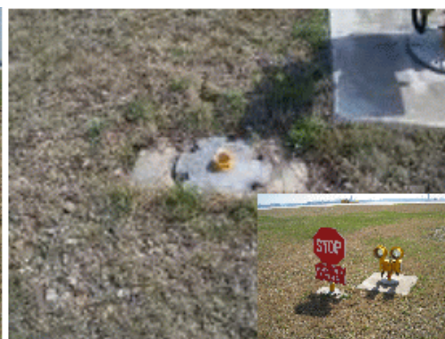
[Photo 9] Stop sign damaged
