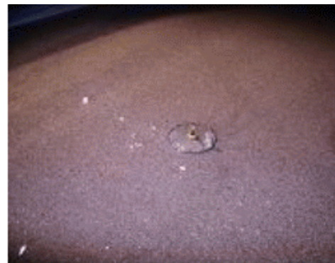
[Photo 7] Runway edge light damaged
