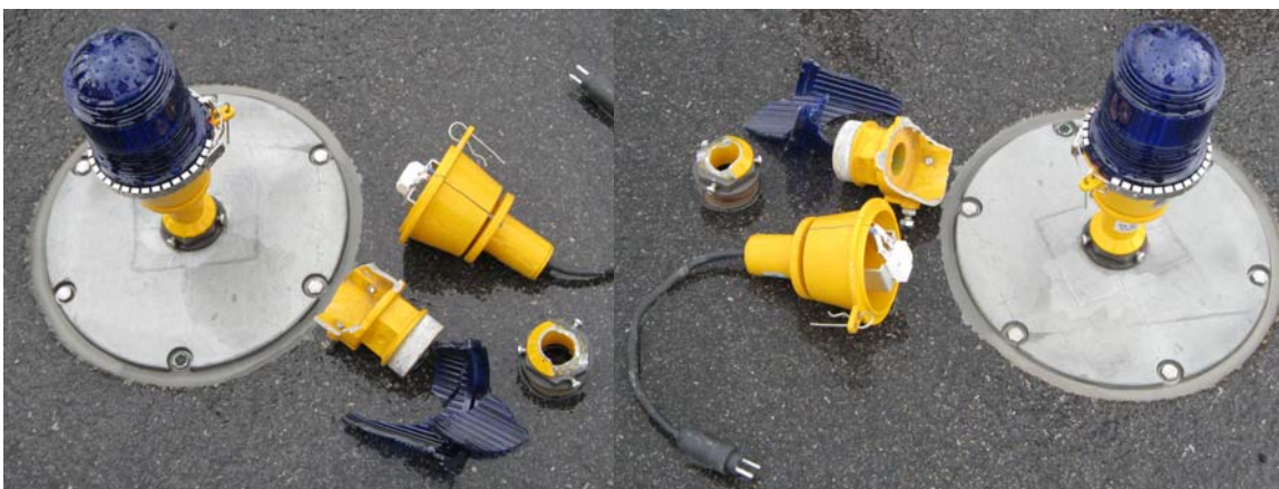
[Photo 7] Taxiway lights damaged and restored to normal condition
