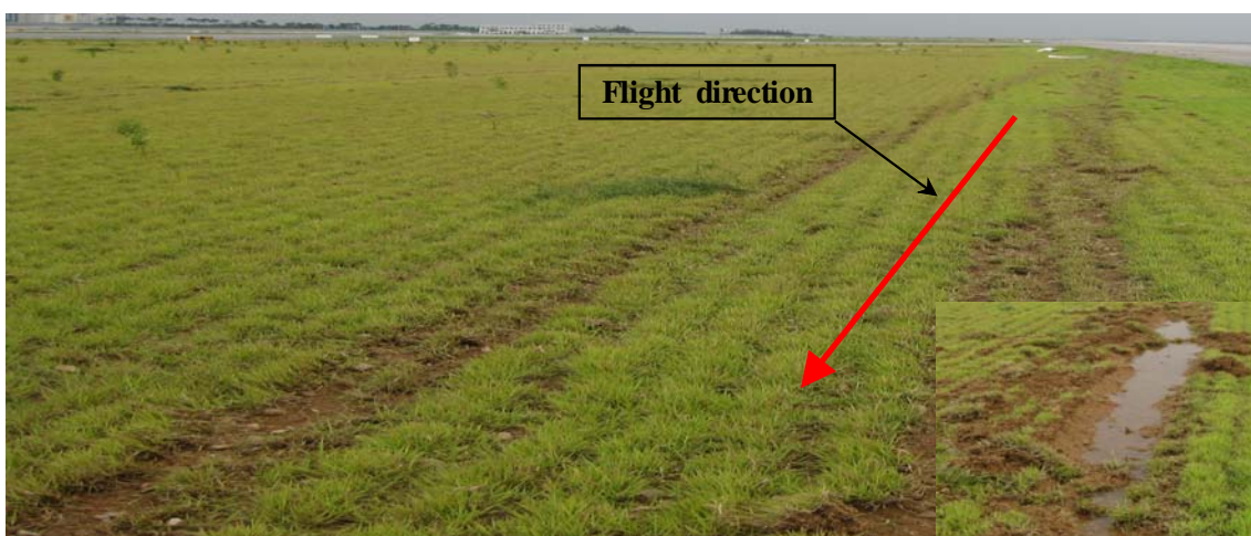
[Photo 9] Landing strip damaged
