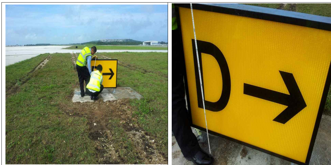
[Figure 13] Airport Facilities Damage
